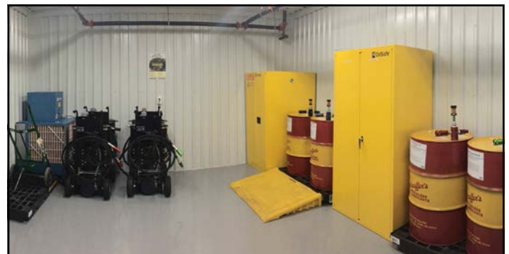
After: Lubrication storage facility
